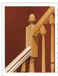
Handrail runs straight into the top block of the newel post at all landings.
